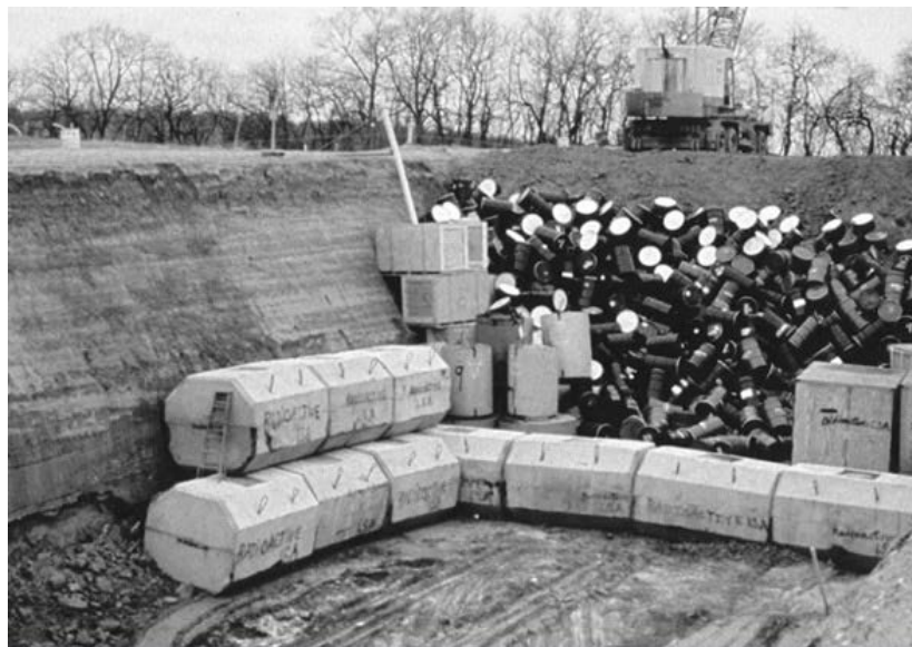
Figure C-33. Sheffield, IL Unlined Trench Burial of Waste during 1960s
